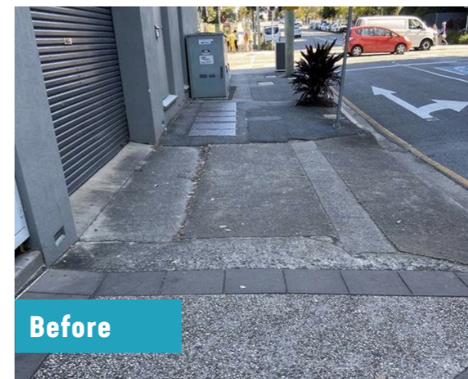
Uneven and narrow walkways, with different footpath treatment in each section.
